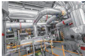
Heat exchange pipes of the thermoelectric power plant
