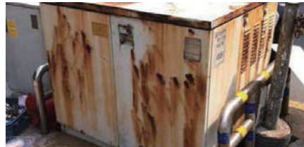
Before removing the rust
